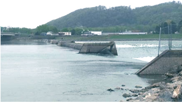
Figure 5-3 | One section of an inflatable dam, not inflated
